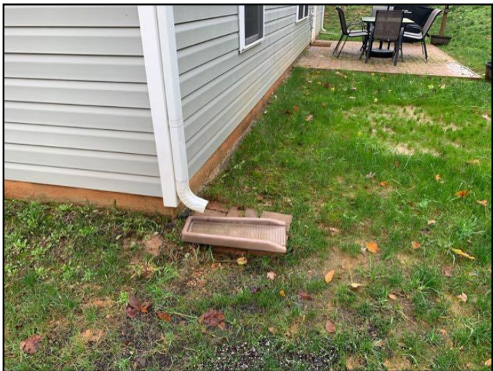
Discharge too close to building
