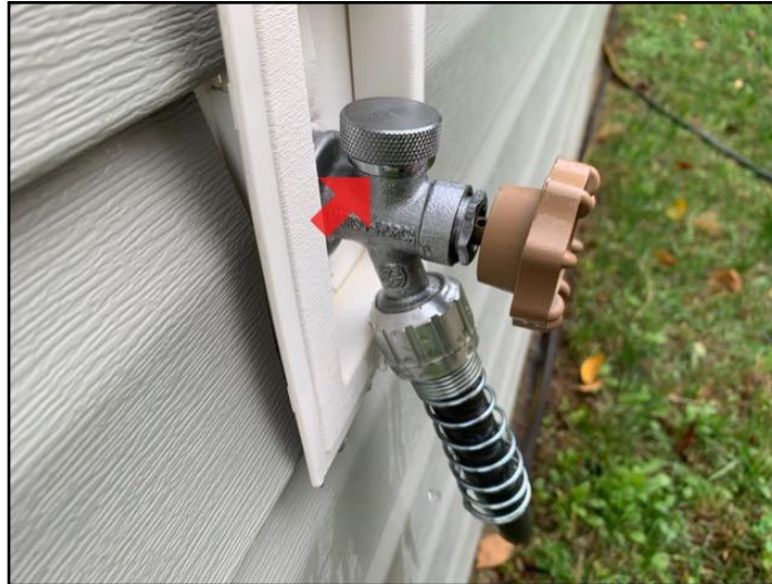
Backflow prevention defective
