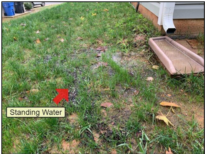
Improper slope or drainage
