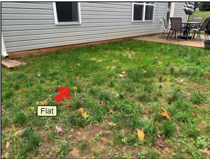
Improper slope or drainage
