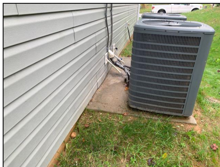
Too close to grade
